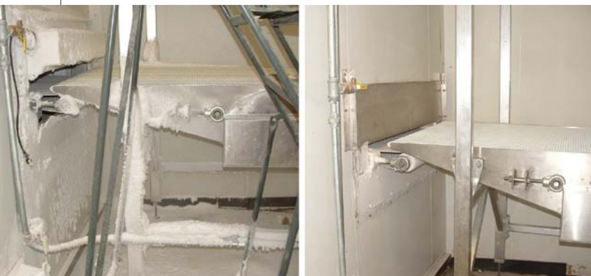
▶ (Left): At Orlando Baking Company, ice and snow built up on freezer coils, the opening to the freezer, the floor and the equipment. (Right): After installing IJ White’s Auto Pressurization System and establishing proper airflow, the ice and snow problems vanished from equipment and the freezer space. Source: IJ White.
