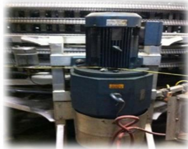
Main Drive Gearbox
